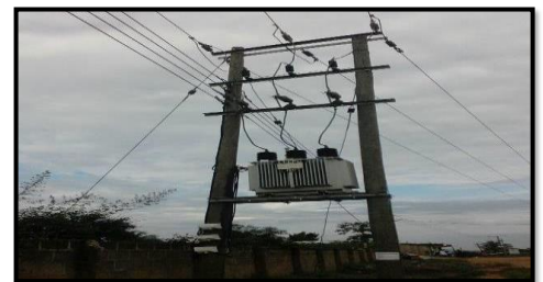
Fig 20: Pole mounted Transformer
